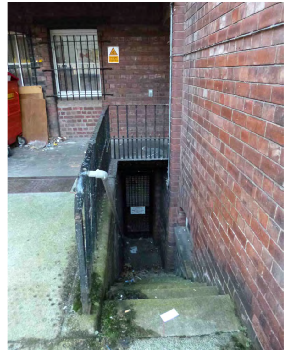
Access stair down to lower ground level of the North Annex, entering under the Post Office
