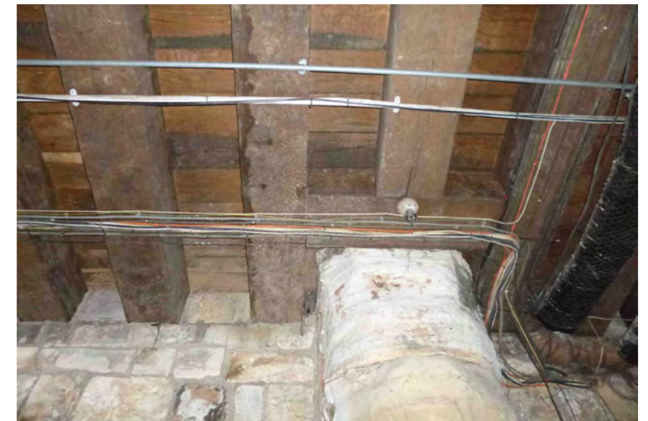
The Guildhall floor construction over Common Hall Lane comprises closely spaced oak beams that support 44mm oak boards
