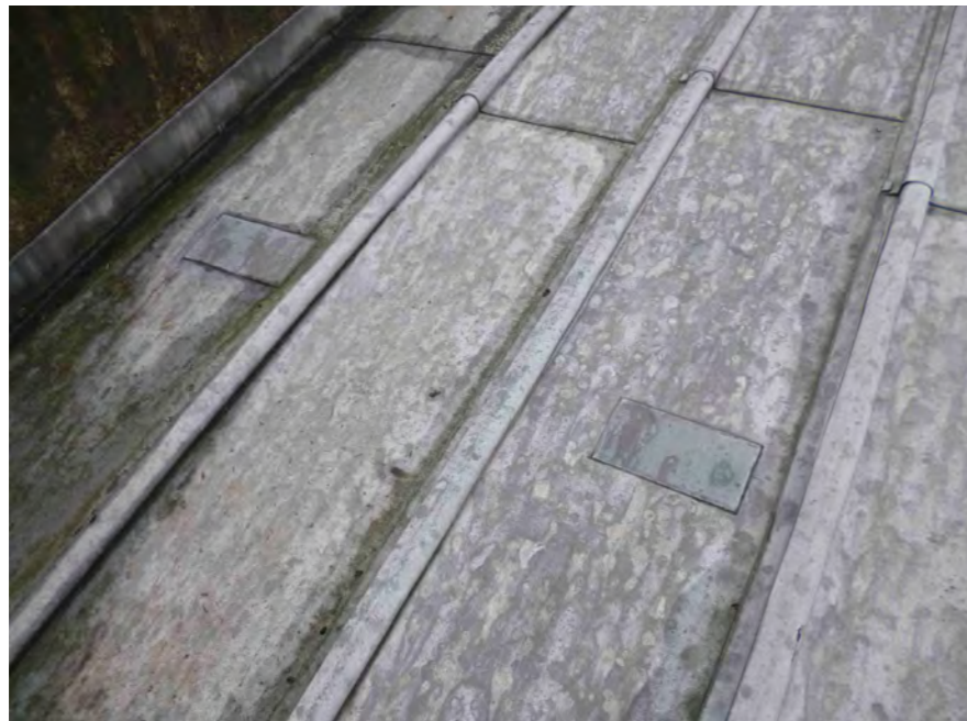
Various patch repairs where the lead has corroded through from below
