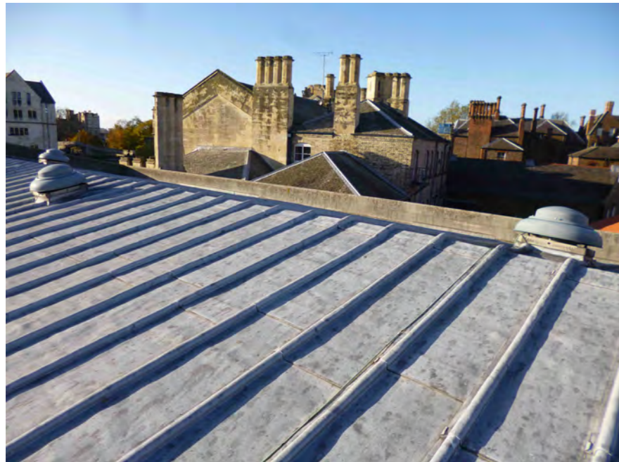
Three ventilators have been installed to try to dry out the roof construction
