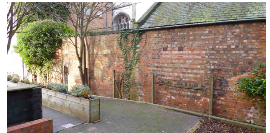
Three visible bricked-up windows in the south wall of the South Range facing the Cineplex
