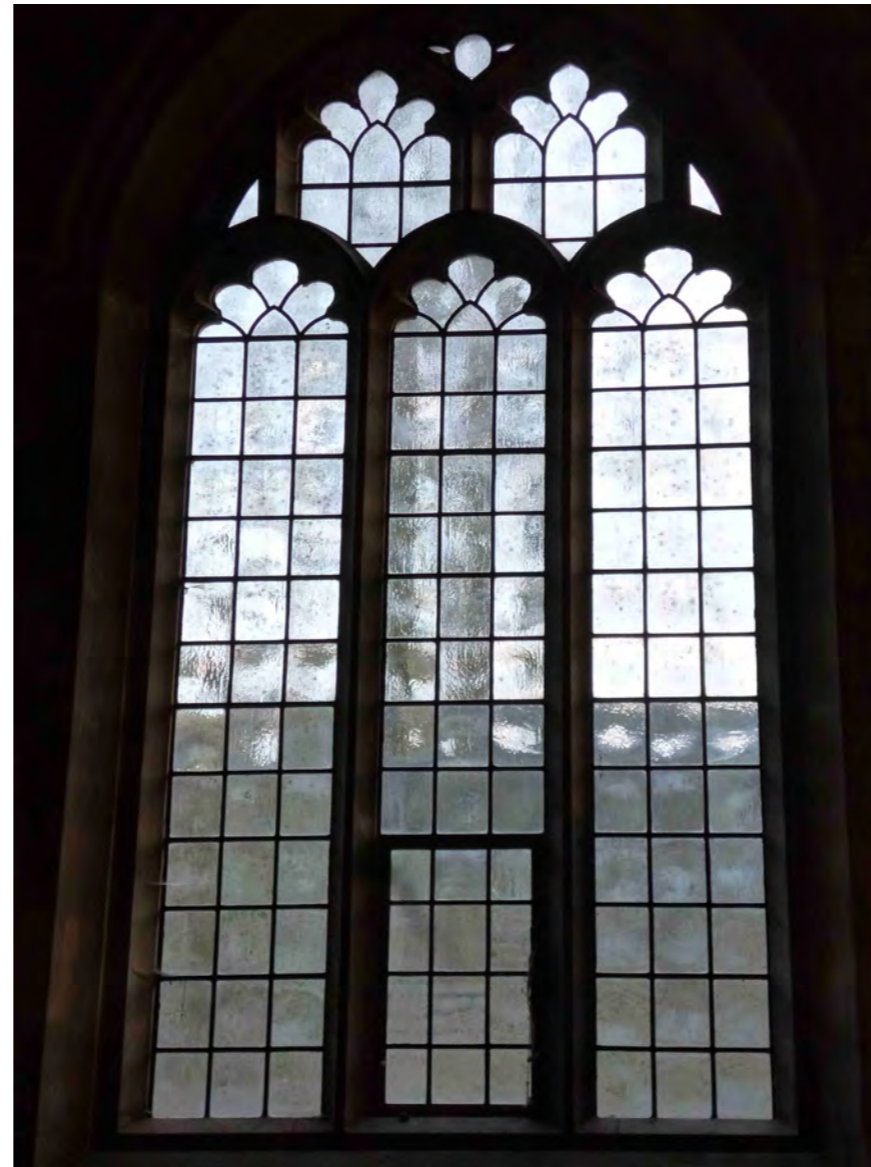
Overall view of a typical window. There are 10 of this type out of a total of 13 windows.
