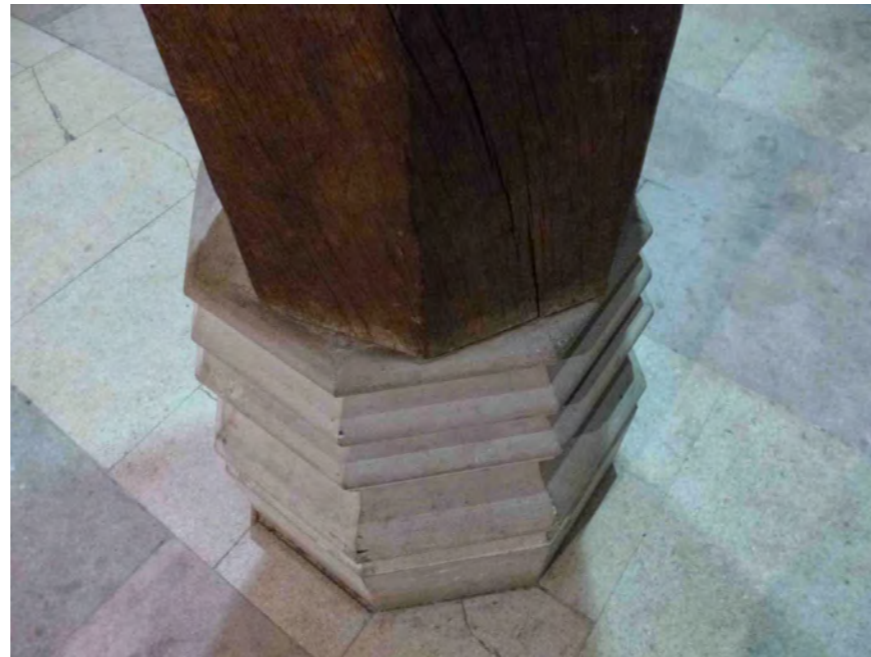
The base of a timber column in the Guildhall showing severe twisting and movement
