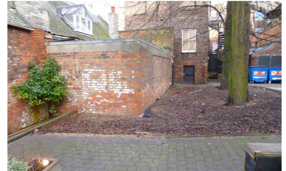
There is an apparent flying freehold above the single storey extension
