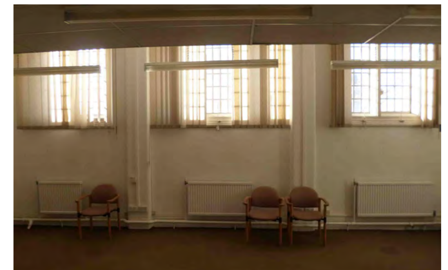
The high windows on the first floor of the riverfront block of the North Annex
