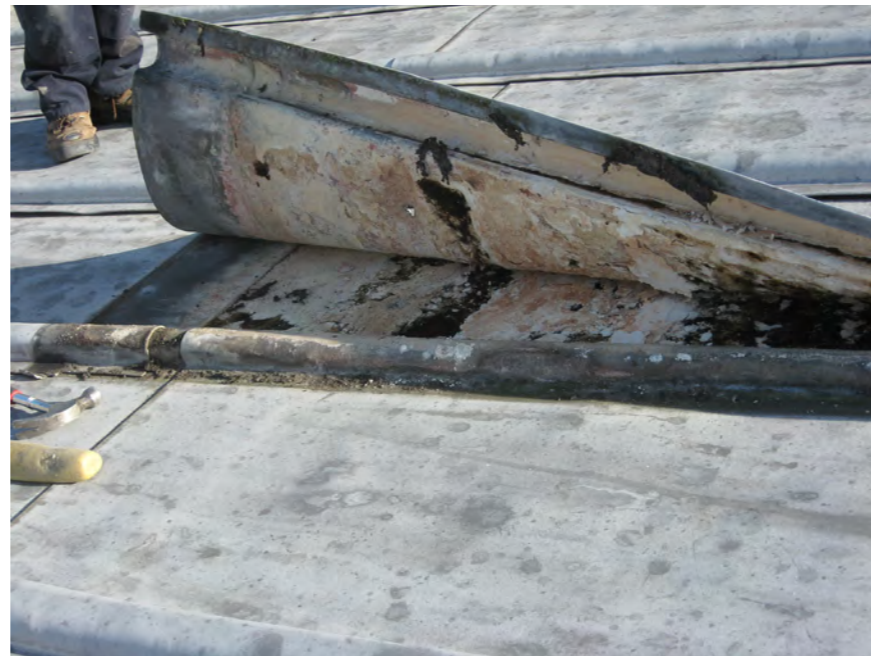
Investigation in 2005 revealed significant carbonation under the ledge sheeting (photo Steve Owen)
